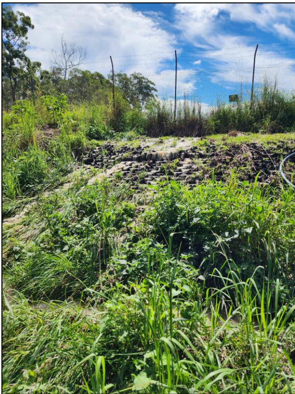
Figure 3: Back of Sediment Dam (S7) overflowing and discharging to surface water bodies downgradient ( 8 April 2024)
