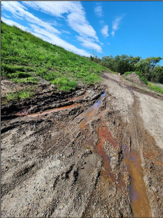
Figure 3: Figure 1: Potential Leachate migrating from capped landfill area - south east of the leachate dam (8 April 2024)
