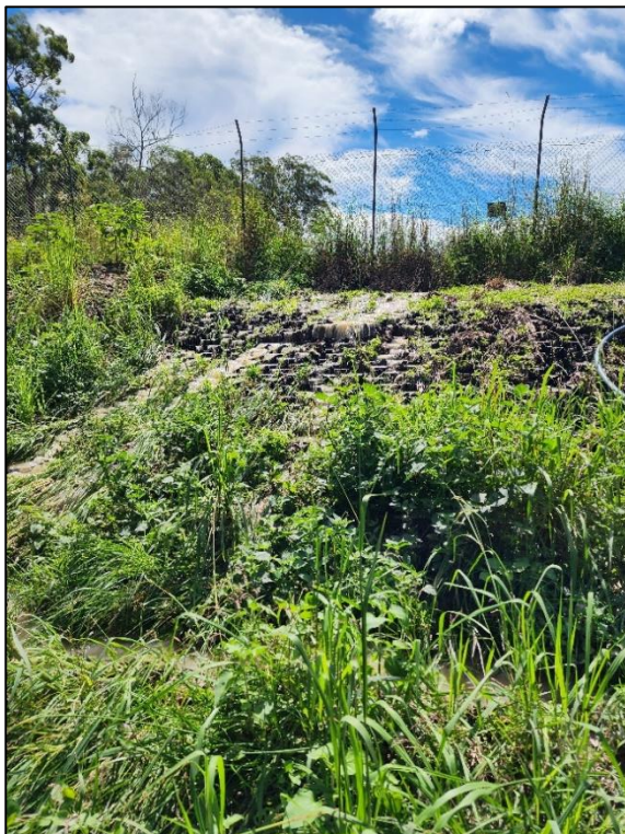
Figure 5: Overflow of Sediment Dam (S7) ( 8 April 2024)
