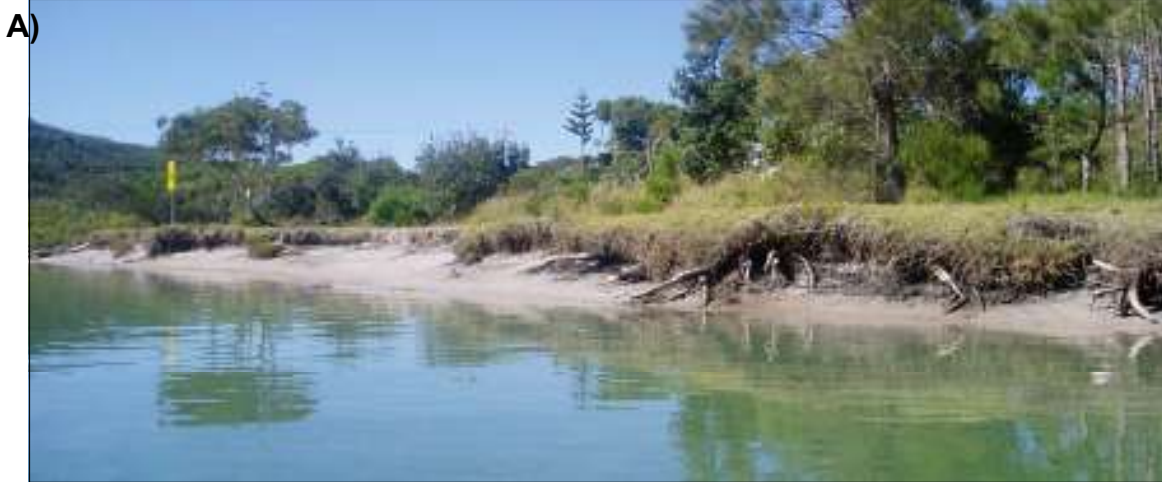
Plate 4 Typical example of moderate bank erosion in the Marine Tidal Delta Process Zone A) slab type block failure and slumping. Note sandy soils, poor vegetation cover and evidence of undercut and dead tree roots in bank.
