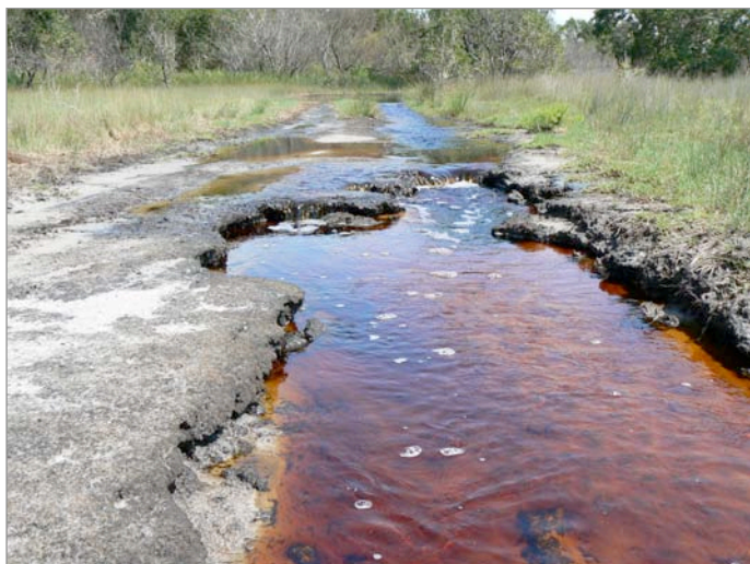
Plate 6 Foreshore erosion caused by vehicle tracks concentrating stormwater runoff
