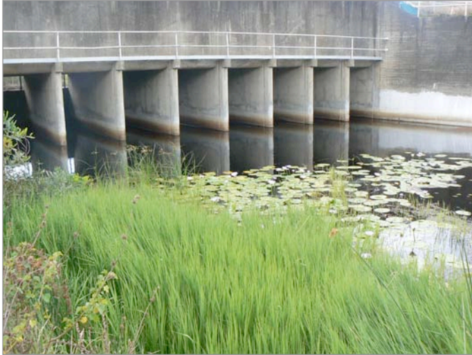
Plate 1 The Korogoro Cut floodgates which operate between the Swanpool and Korogoro Creek.
