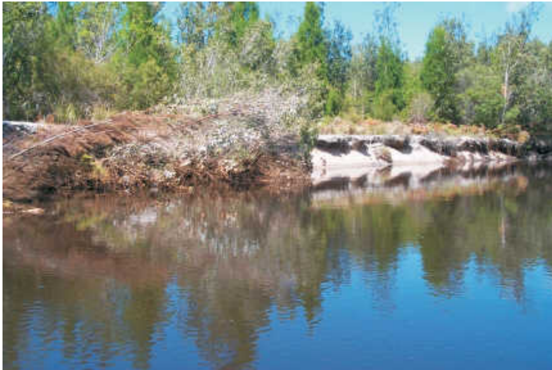
Erosion along the creek downstream of the flood drain
