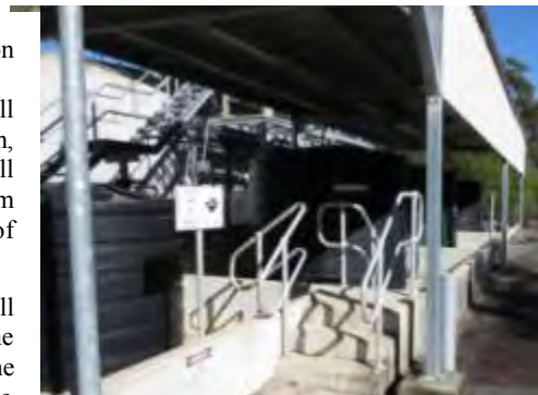
Chemical tanks at Hat Head STP
