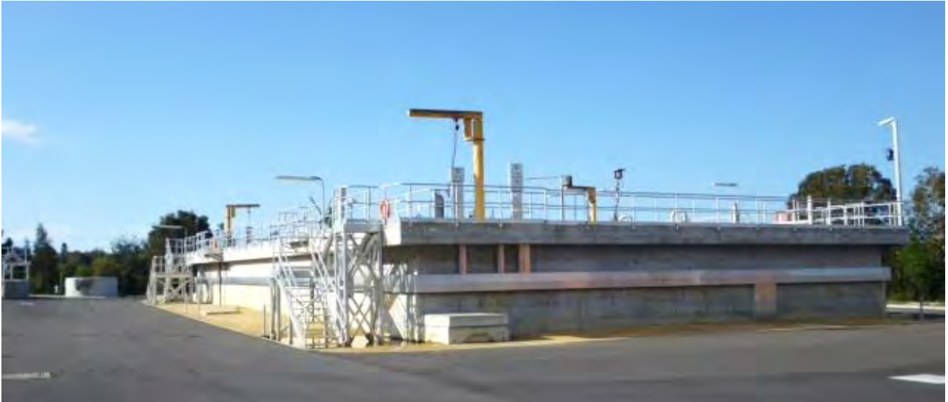
In 2009 at South West Rocks Sewer Treatment Plant, the existing 3 pasveer channels were supplemented with a dual tank sequential batch reactor
