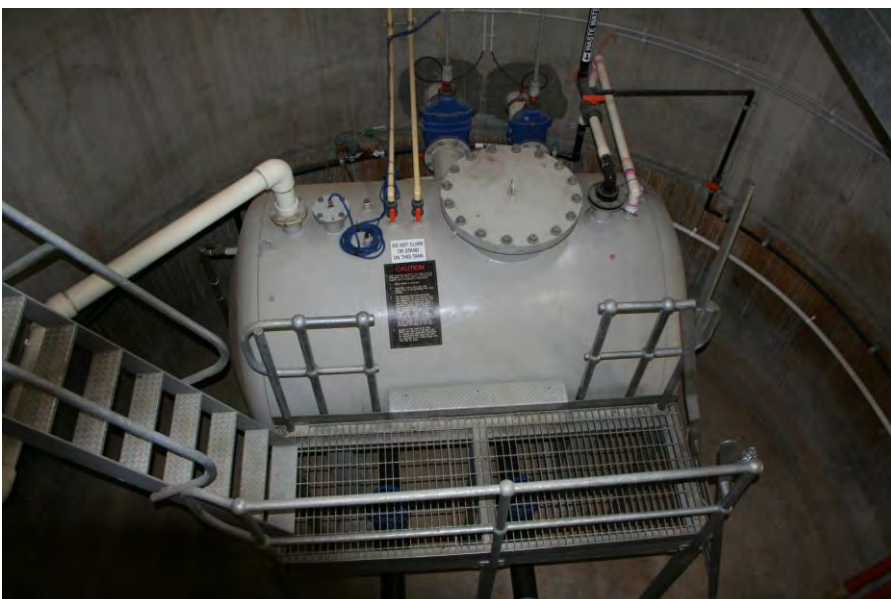
Vacuum tank at Hat Head HI pump station
