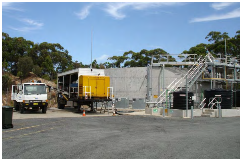
Mobile centrifuge dewatering the sludge at Hat Head STP
