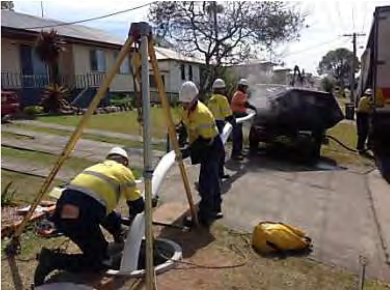
Relining a sewer main in West Kempsey. The mains are first checked with CCTV camera, cleared of roots and jetted with water until the pipe is sufficiently cleaned. The line is then re-camered and the new internal lining pipe is inserted inside the old pipe and lastly new junctions are inserted. Finally the mains are re-camered to ensure workmanship is satisfactory
