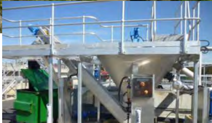
New grit removal system
