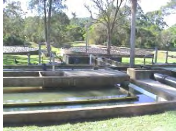
Sedimentation tanks & trickling filters
