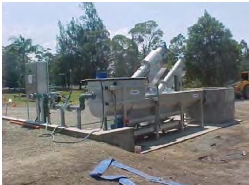
The septic receival unit at South Kempsey STP is designed to pre-treat septic waste prior to further processing at the sewage treatment plant
