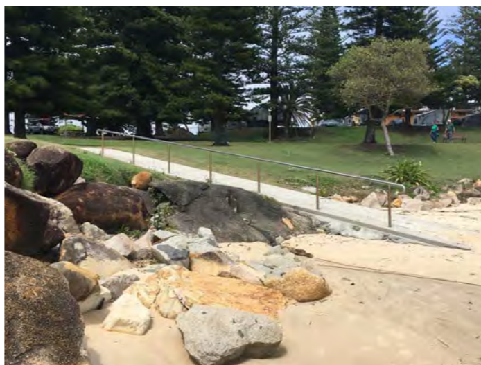
Existing access ramp to the beach non compliant- improved access to be investigated
