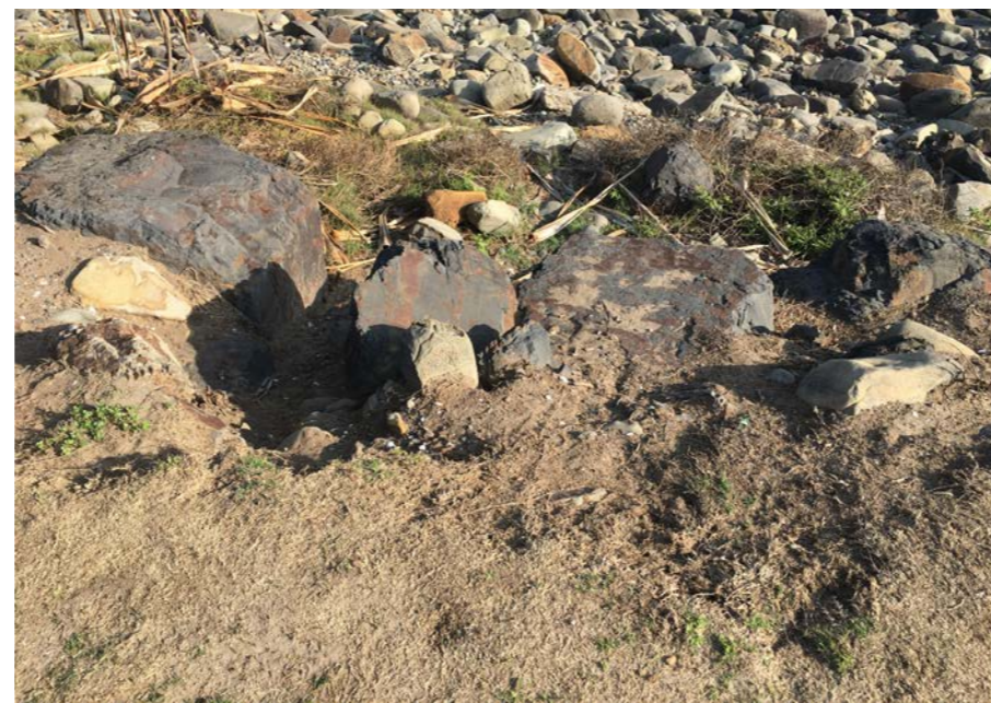
Tracking and erosion along edge of sea wall
