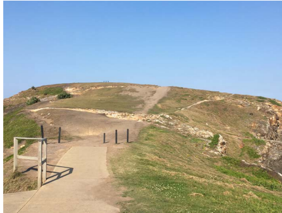
Tracking and erosion on Little Nobby
