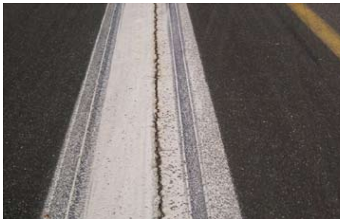
Cracking on bitumen runway
